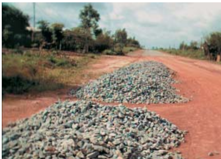
Sugar cane development project in Tay Ninh province, building a secondary road – Photo OG – AfD
